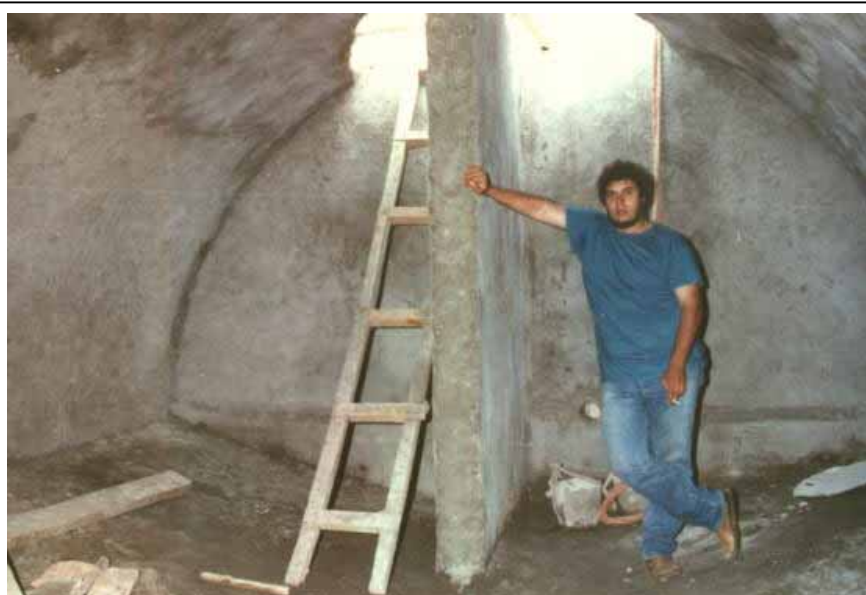
View in a canal digester, Burundi
