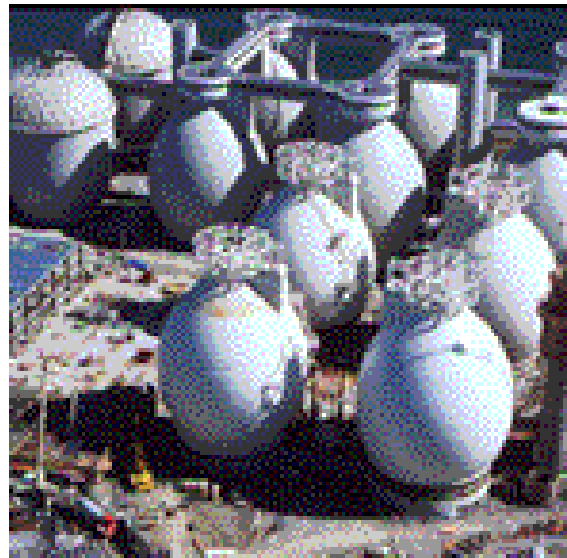
Fig. 7: Egg-shaped reactors for anaerobic sludge digestion (Source: TBW)
