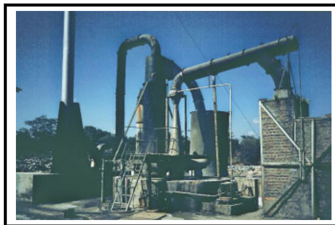
Fig. 7: Off-gas cleaning system of a lead recycling furnace in Zimbabwe
